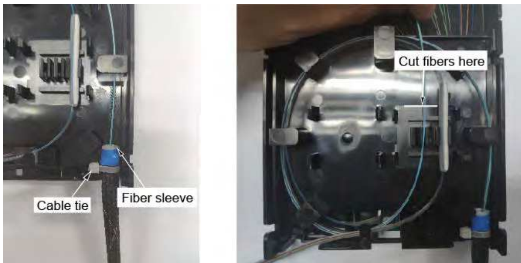
Figure 5. Secure Incoming Cable
