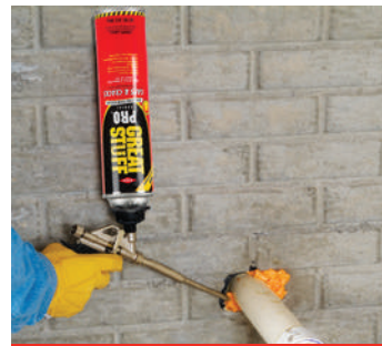
Plumbing and pipe penetrations
